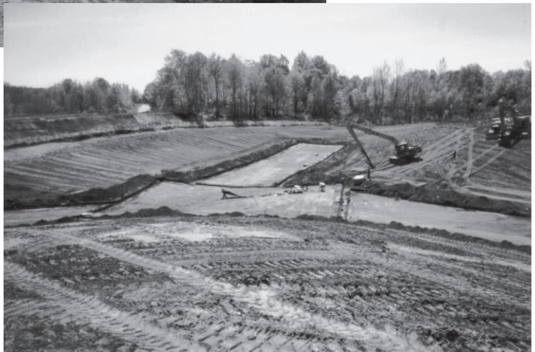
(To the right) Water will be collected at the lowest point of the reconfigured Tar Lake to prevent seepage and allow evaporation. Vegetation along the gradually sloped walls of the former deep pit will also control moisture.
