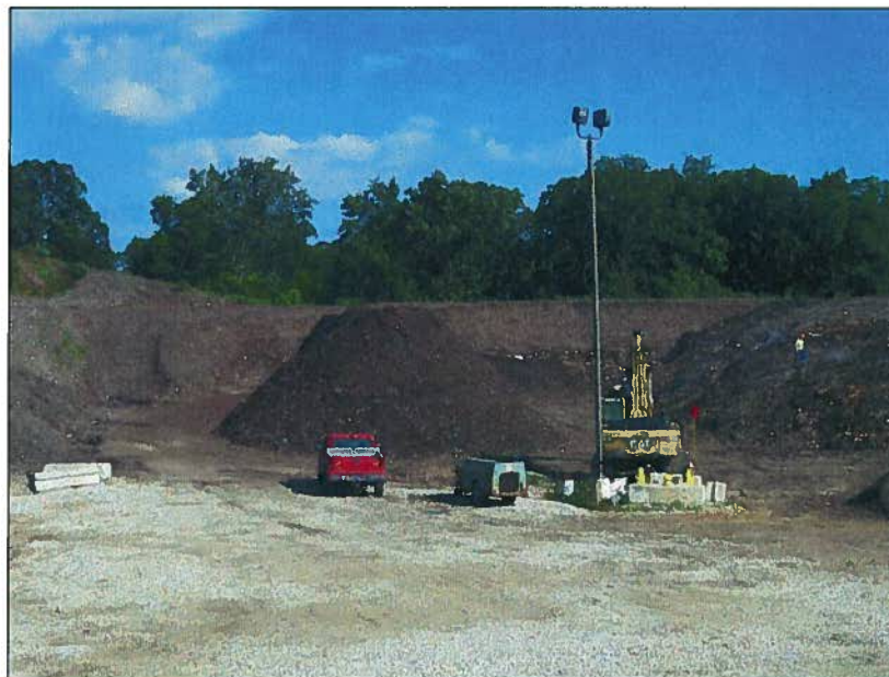
Photo 2. VIM Recycling, Elkhart operations Description: Progress of removal on west side of C-Pile Date Taken: 9/18/09
