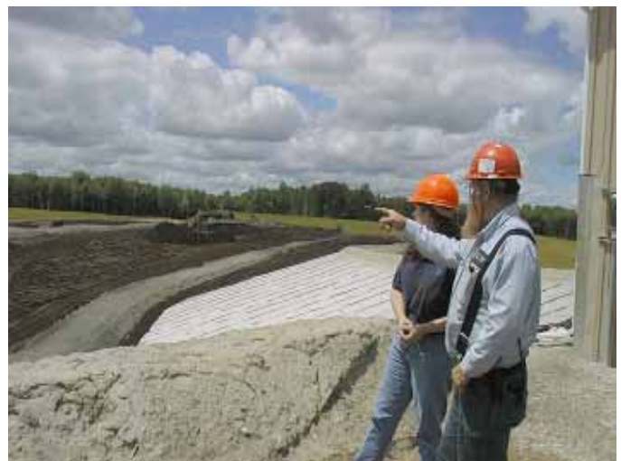
Terese Van Donsel, U.S.EPA's remedial project manager, and Mike Cole, site foreman, discuss the placement of Superfund material in the Millennium landfill.
