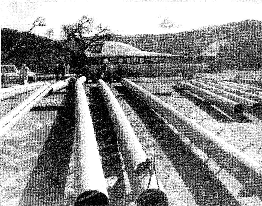
Tubular steel poles, specially designed to support the SLAC power line, about to be placed by helicopter to avoid site damage
